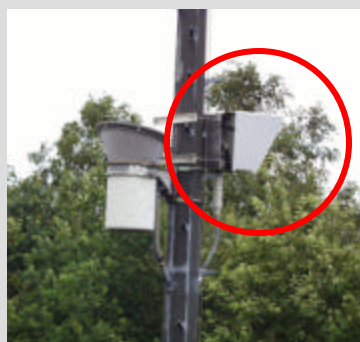
Basestation Antenna Transrapid, 38 GHz
